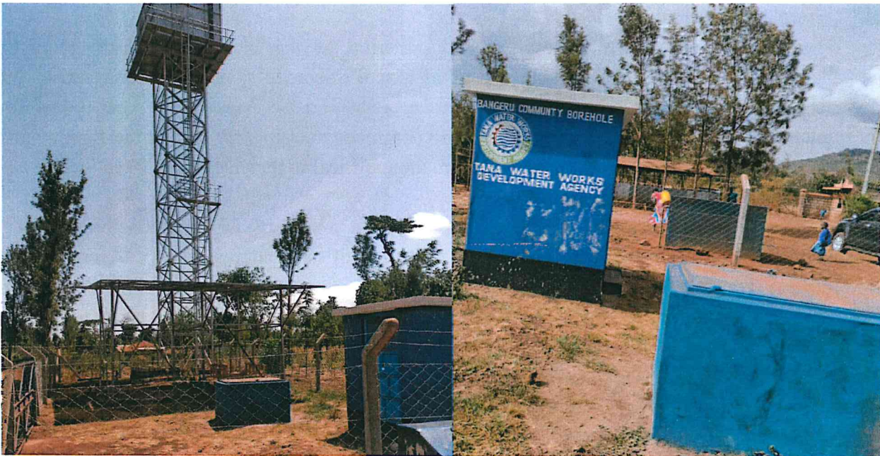
Figure 10: 48m 3 Elevated steel tank and pump house at Bangeru Community Agithi borehole with a yield of 36m 3 /day in Kianjai, Meru County
