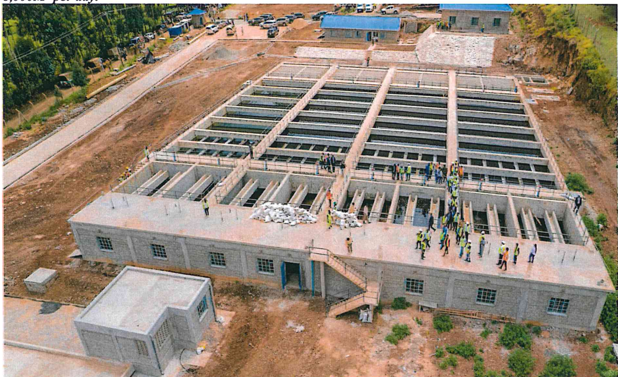
Figure 2: Ongoing works of the sedimentation basin at Muratiri Treatment Plant – Kerugoya-Kutus Water Supply Infrastructure within TWWDA area of jurisdiction. The treatment facility is supposed to treat 30,000m 3 /day of water.
