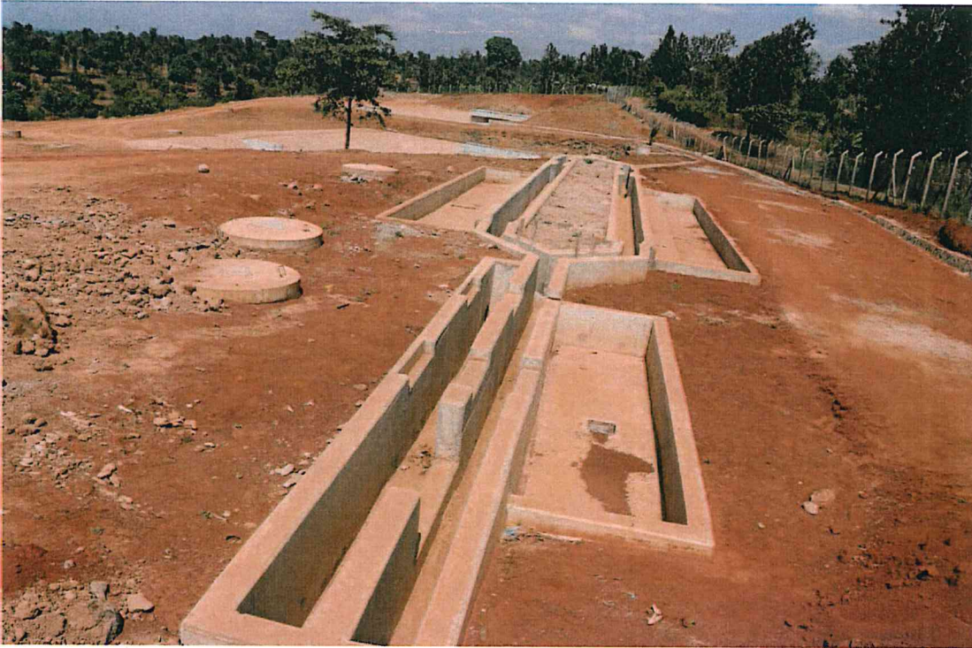
Figure 7: Inlet works at Chogoria Sewerage Infrastructure
