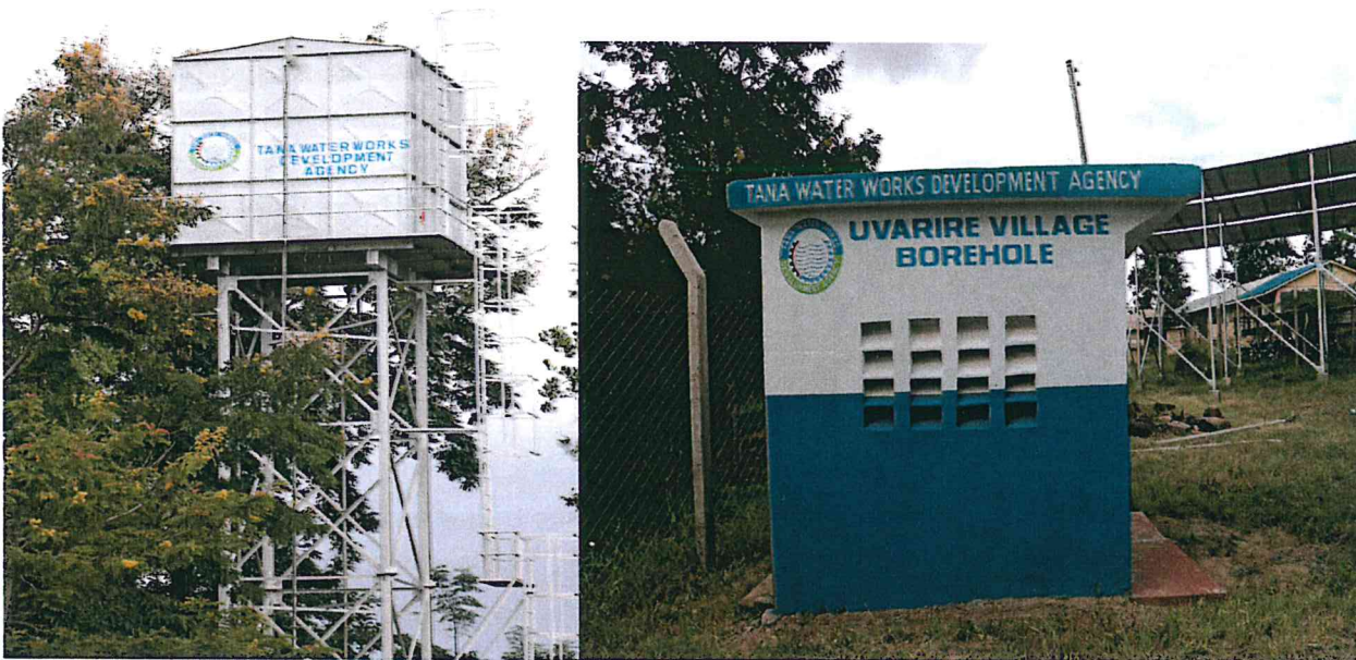
Figure 11: 48m 3 Elevated steel tank and pump house at Uvarire Village borehole with a yield of 12.5m 3 /day in Mbeere, Mbeere Embu County
