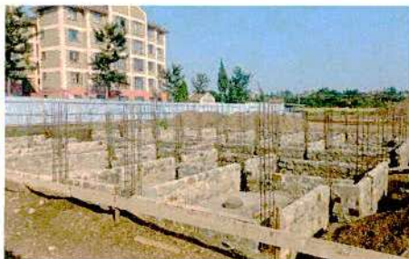
The ongoing works at the Konyakwar Phase III project in Kisumu Town.
