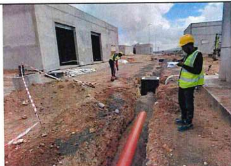
Stormwater process pipes at WTP
