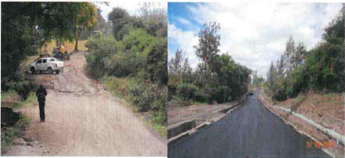
Figure 3: Maragoli Road in Nakuru county before and during upgrade under Low Volume seal programme
