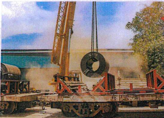
Offloading of hot rolled coils (HRC) at Davki Athi River plant, following the construction of an MGR rail siding to the plant. Railway sidings enable us offer last-mile services to our customers. What are you transporting
