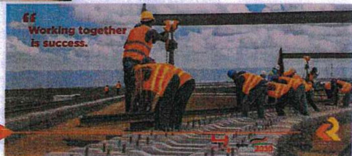
On-going rehabilitation of the rail infrastructure in western Kenya. An efficient rail is an enabler to all regional economies
