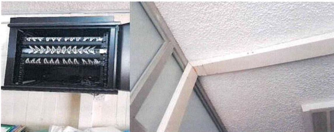
Structured cabling and trunking
