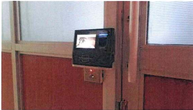
Biometric systems have been installed on all floors including the server room
