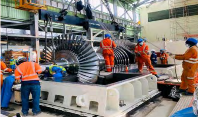
83.3 MW Olkaria Unit 6 turbine rotor assembly
