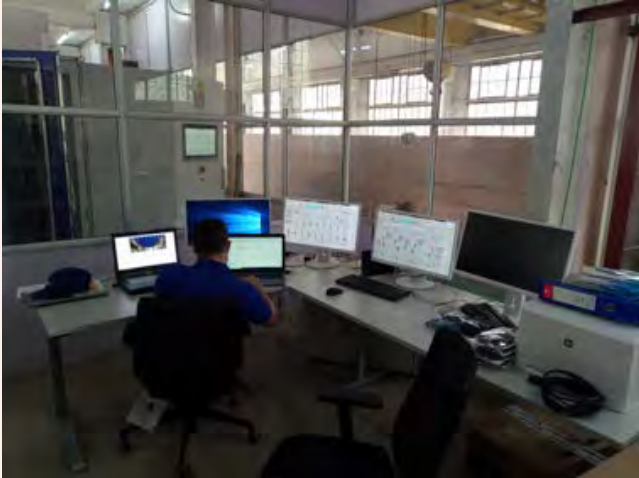
Wanjii Power Station Control Room
