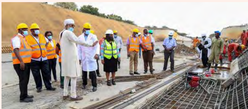
The Masinga spillway repair works being inspected by the Board Chairman, General (Rtd) Samson Mwachethe, other Board Members and Management team
