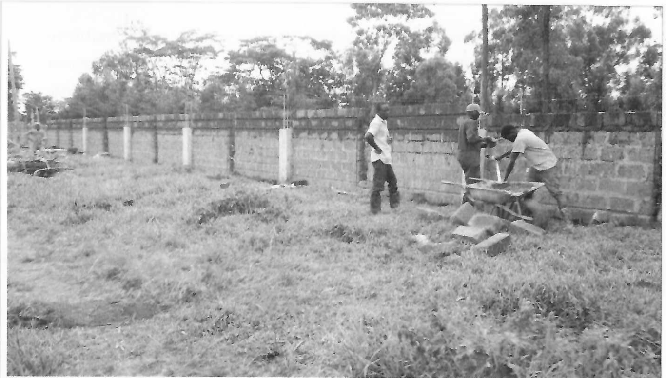
Figure 9: Construction of the College Perimeter wall to enhance security and safety of its property at Ksh 250M.
