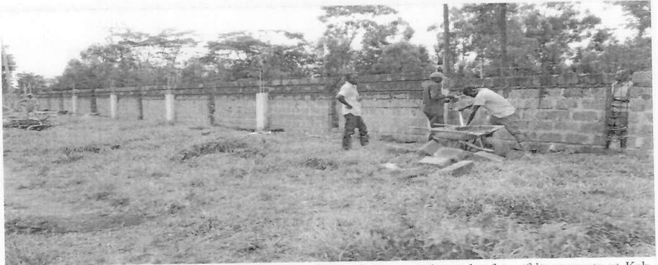
Figure 9: Construction of the College Perimeter wall to enhance security and safety of its property at Ksh 250M.
