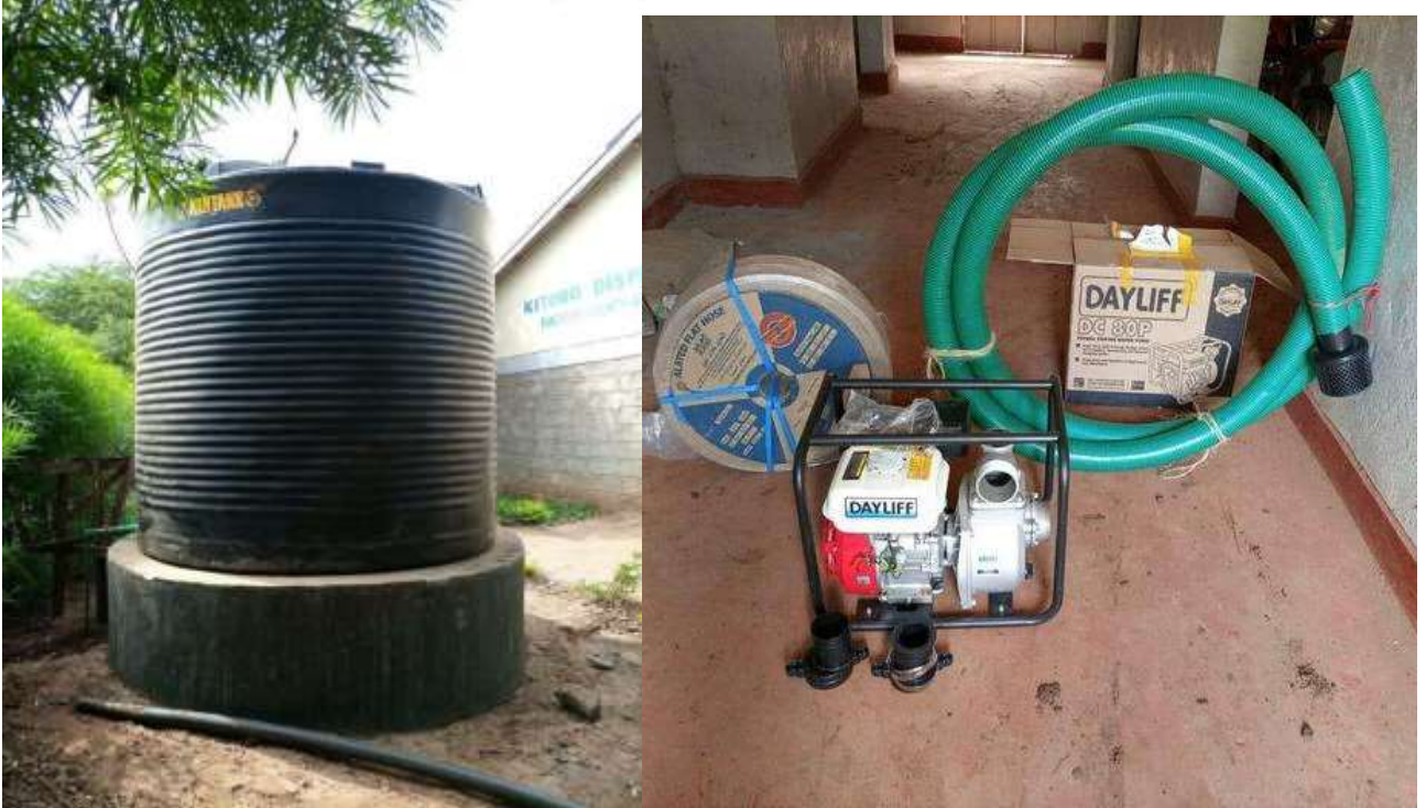
Water tank, pump and pipes to Kitobo Dispensary
