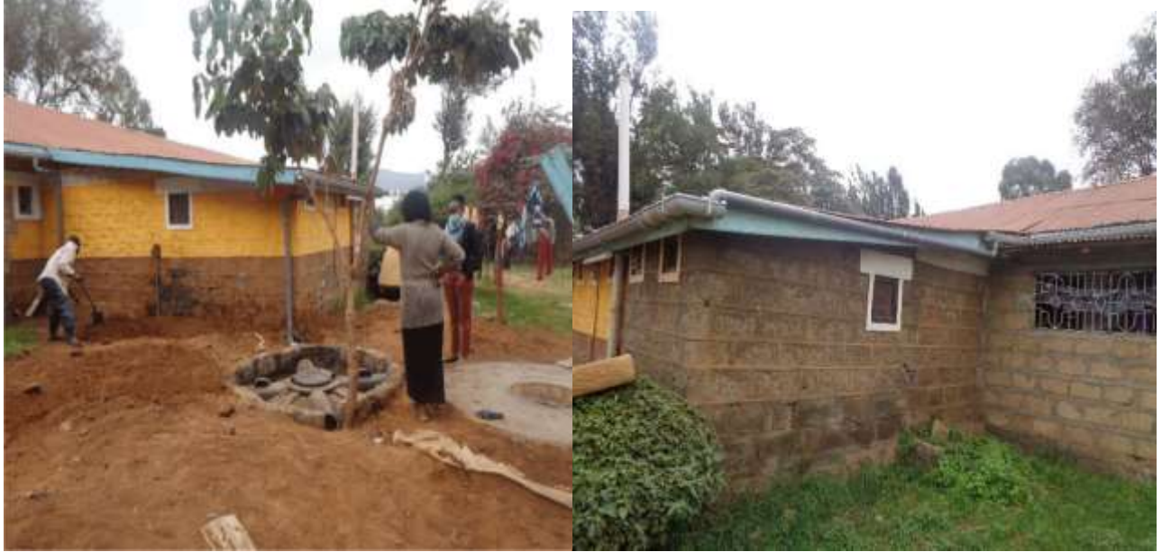
Water tanks and gutters at Mai-Mahiu Children's Home
