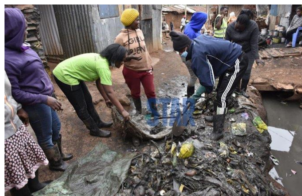
Youth under the Kazi Mtaani programme unblocking the sewage system in Kibera
