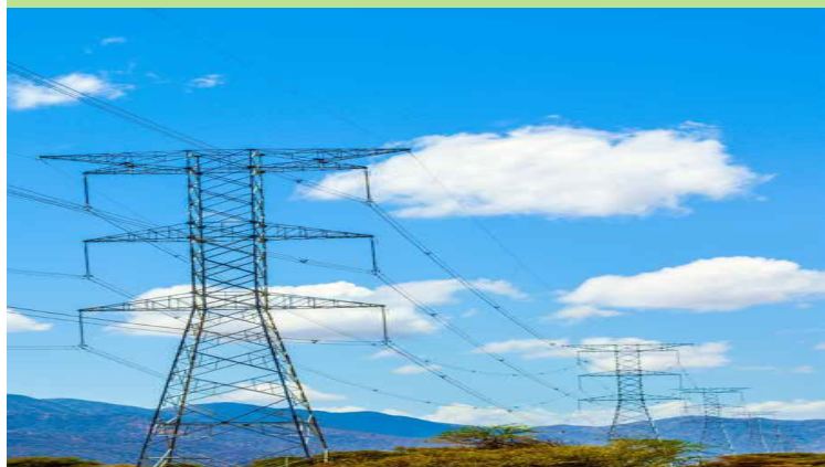
Alternate Power Pylon for Power Transmission
