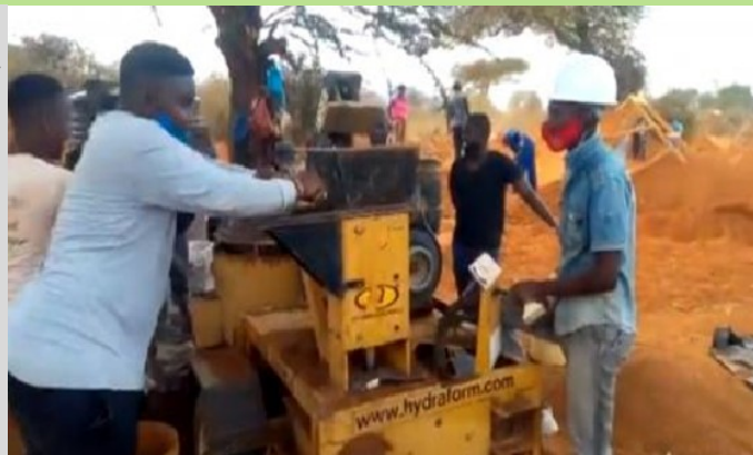
Youth making soil blocks using ISSB technology that will be used to construct 30 additional classrooms at Mikuyuni Secondary School in Kibwezi .
